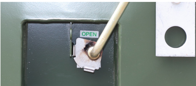
A sturdy operating handle is stored in each operator compartment. The padlocking provisions on the compartment doors accommodate the majority of available padlocks.
